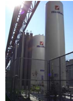
O 2 / CO 2 tanks
